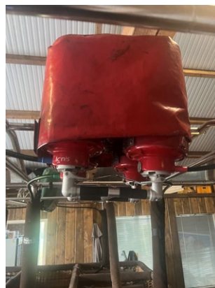
▲ Red transport cover over the red burners. (Source: Pilot)
