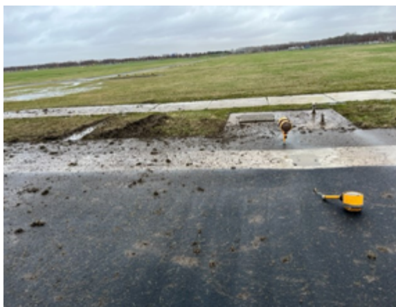
◀ Figure 5: One of the sheared off runway lights. (Source: Amsterdam Airport Schiphol)
