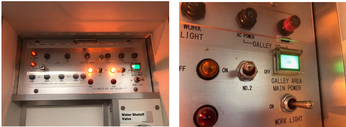
▲ Figure 1: On the right in both pictures, the green lit galley area main power button.
