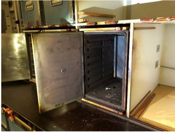
◀ Figure 2: The failed oven.
