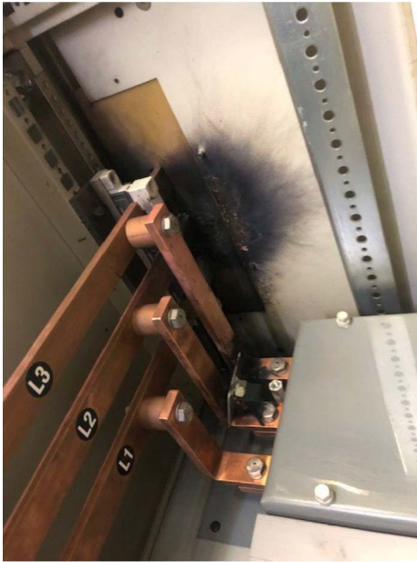
▲ Figure 23 Fire in Switch panel. (Source: MV Jade)
