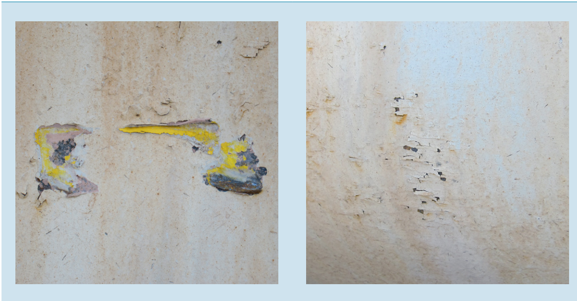
Figure 29: The left-hand photograph shows the mechanical damage observed below the manhole cover on the rear wall of the tank. The damage is the imprint of the draw eye on the front of the passenger train. The right-hand photograph shows local crackling of the paint layer on the tank. (Photos: Dutch Safety Board)
