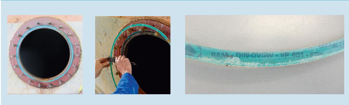
Figure 32: These photographs show the gasket. On the left-hand photograph the (green) gasket is still in the intended flange groove. On the right-hand photograph we see the markings. (Photos: Dutch Safety Board)
