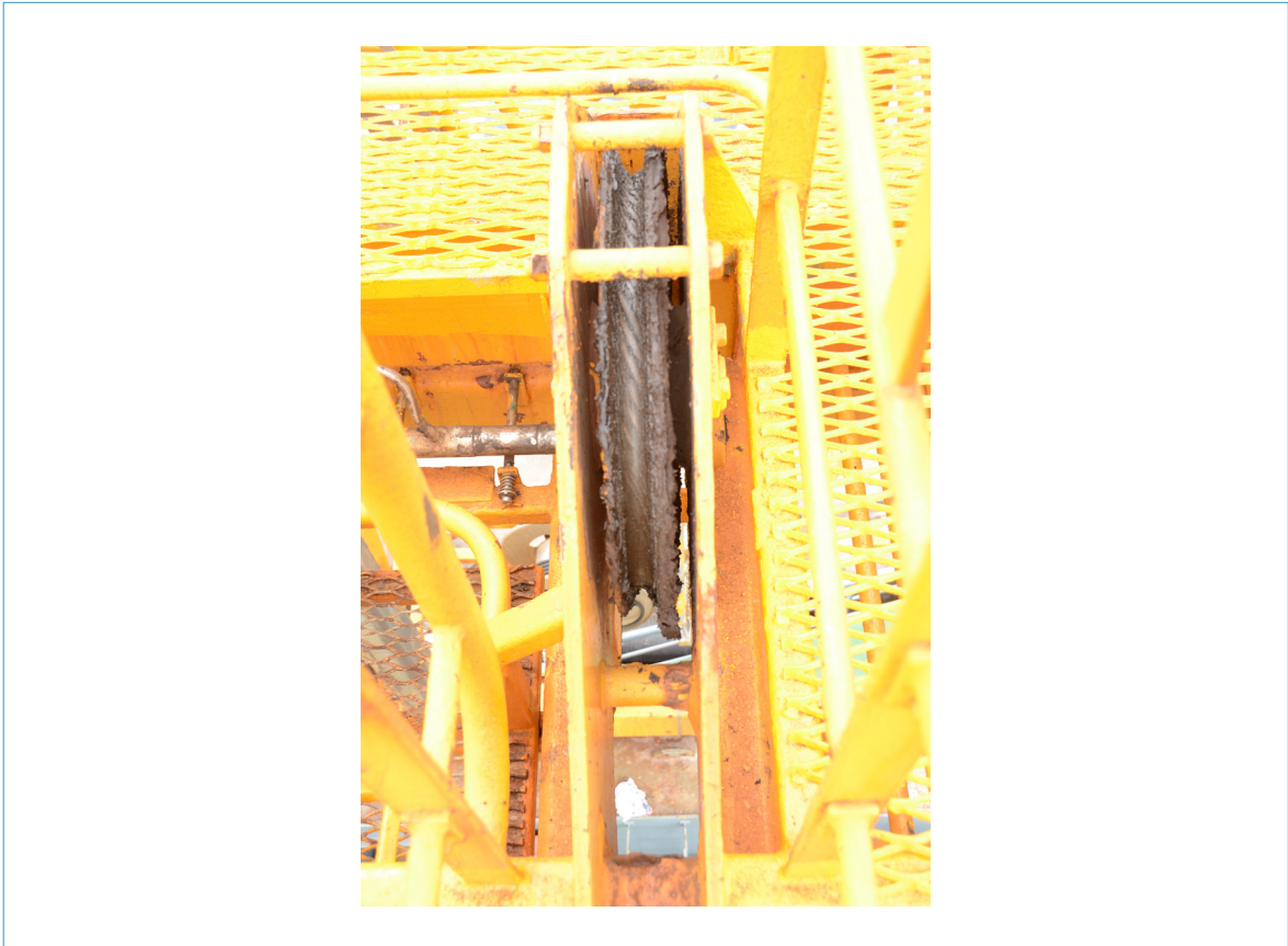
Figure 8: Hoisting cable guidewheel on hatch crane. (Source: National Police)
