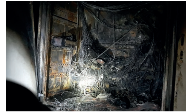
Damage following fire in engine room. (Source: Ship operator)
