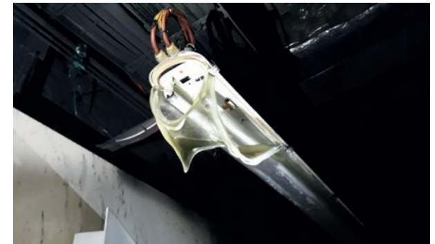
Damage following fire in engine room. (Source: Ship operator)
