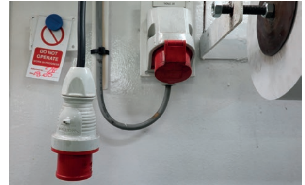
0.9 Kw connection used for the electrical winch. (Source: Dutch Safety Board)
