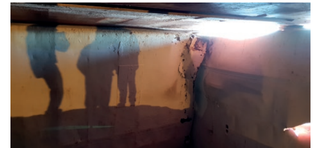
Damage in the hold of the Eems Cobalt. (Source: Dutch Safety Board)
