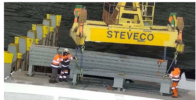
▲ The support beam is hooked to the spreader with two hooks. The two loose hooks can also be seen. (Source: CCTV Steveco)
