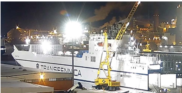
▲ The quay crane being used to move the support beams just before the accident. (Source: CCTV Steveco)
