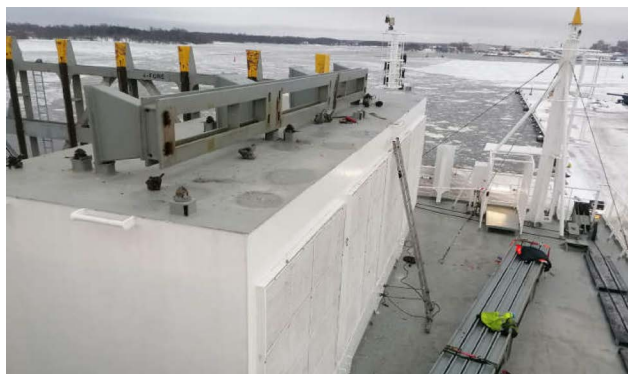
▲ Toppled support beam on housing of ventilator and support beams that fell down on lower deck next to housing of ventilator. Next to this is the loosely placed ladder used by people to climb up the housing of ventilator. (Source: Spliethoff)
