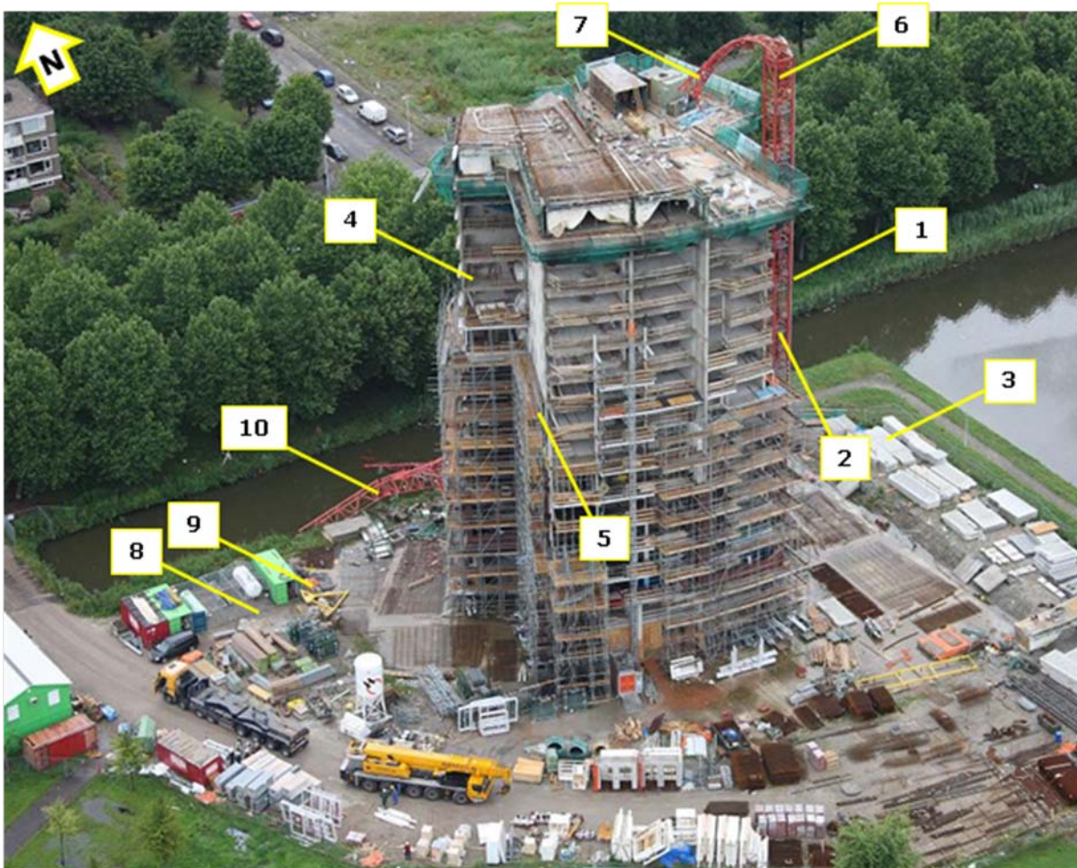
Figure 5 – Overview photo of the construction after the collapse of the crane (source: KLPD Dienst Luchtvaart)
