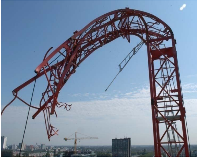
Figure 7 - Bent, broken and torn mast (Photo: Rotterdam Rijnmond police department)
