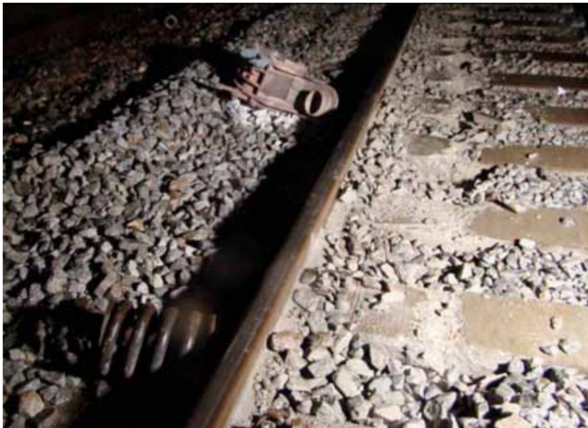
Figure 13: This photo shows the damage the left-hand wheel of the derailed wheel set caused to the concrete sleepers. The overheated axle box and one of the four springs accompanying the axle box lie next to the rail.
