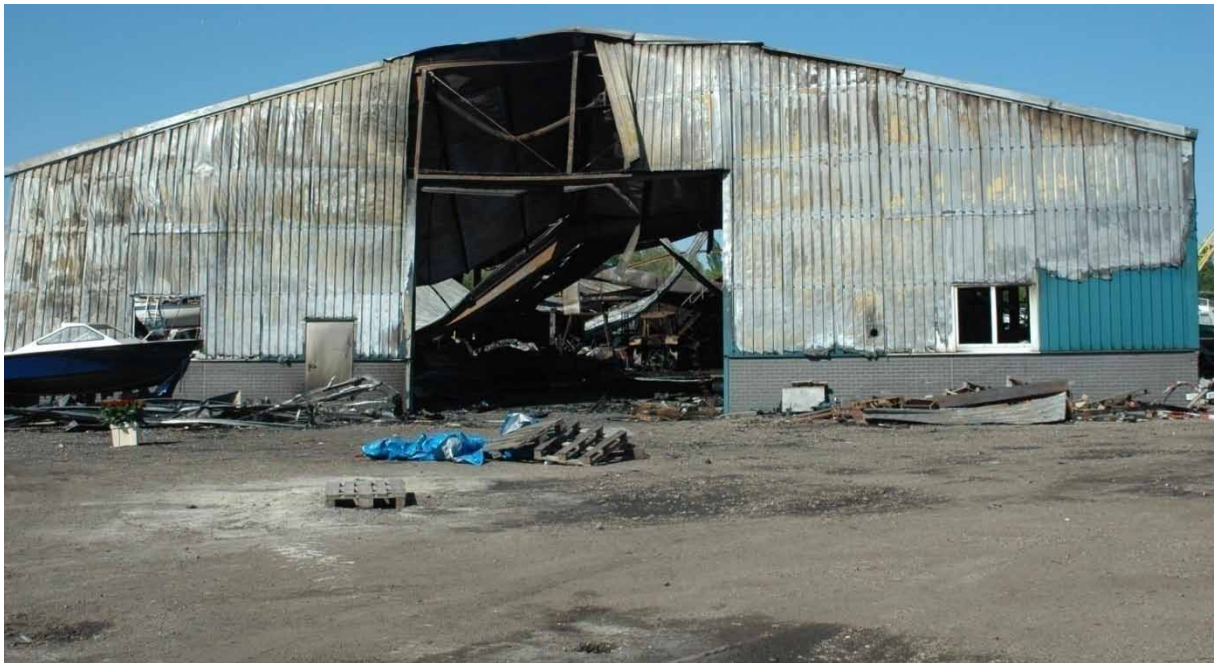
Photograph 2 Front of the shed after the fire. The hole above the door opening was created at the time of the sudden fire spread when part of the front was blown out.
