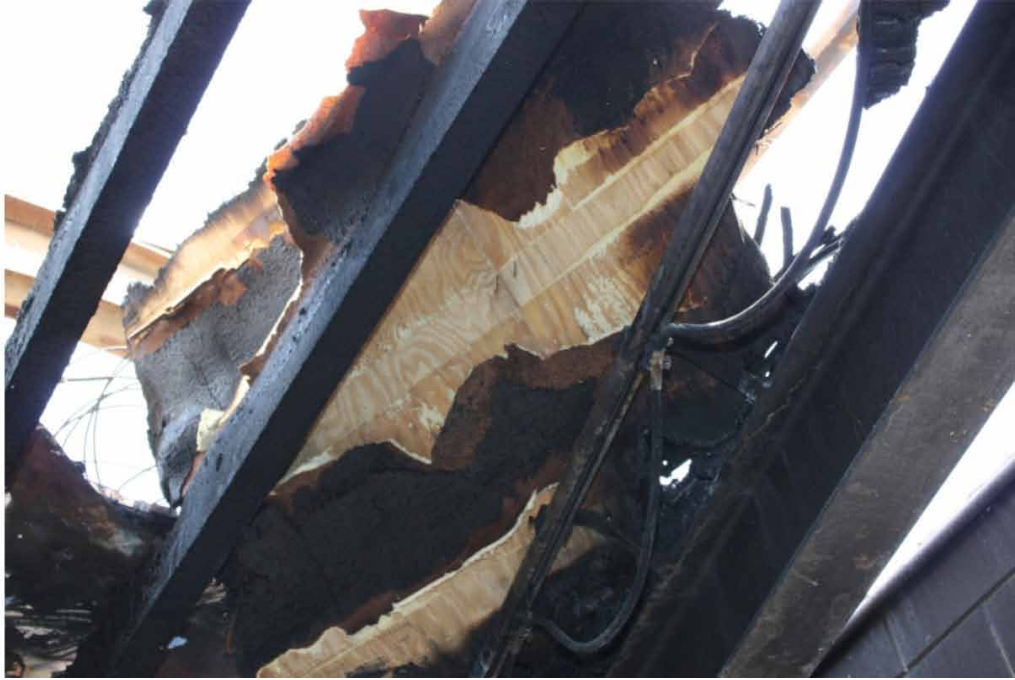
Photograph 6 Engine workshop – thermal attack from attic to workshop
