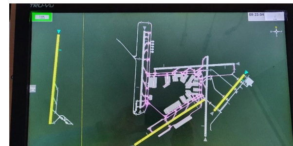
The Airfield Lighting Control and Monitoring System (ALCMS) control panel at Amsterdam Airport Schiphol. The runways illuminated in yellow are available to air traffic control. The runways in grey are unavailable.
