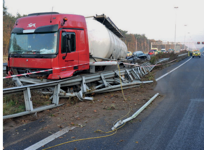
On the A58 near Oirschot a truck swerved as a result of a tyre blowout and drove through the median barrier Source: Police
