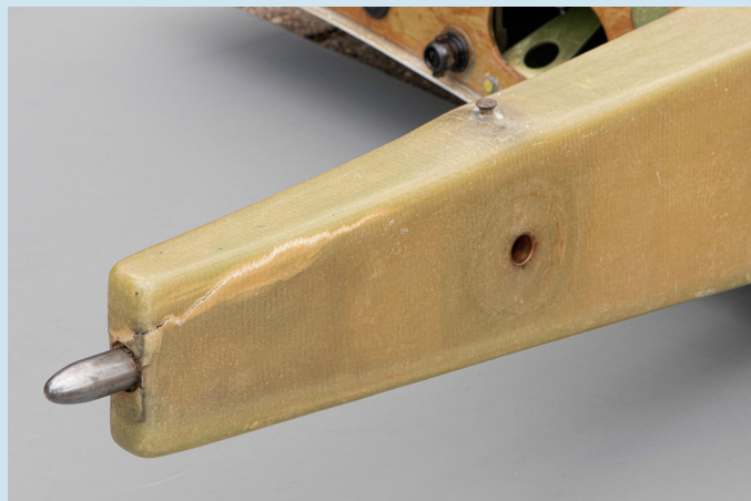
Figure 1: Failed spar of the left wing observed from the leading edge side. (Photo: NLR)
