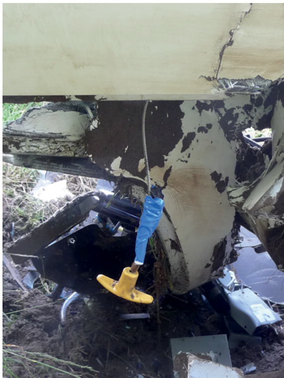
Figure 6: The temporary repair of the molded sleeve, as found at the accident site. (Source: Dutch Safety Board)
