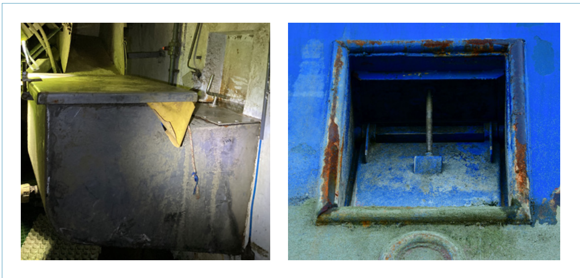
Figure 4: Fish waste discharge chute - side view.
