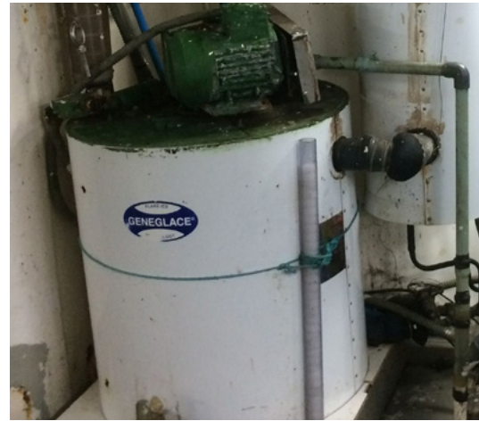
Figure 29: Original freezer installation. (Source: Maaskant Shipyards Stellendam)
