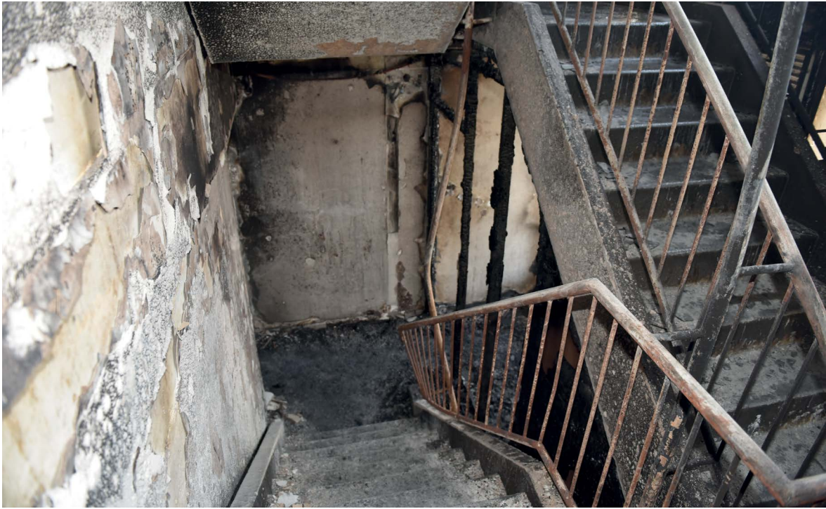
Figure 8: Picture taken from the landings between the ground floor and the first floor (Source: Veiligheids- en Gezondheidsregio Gelderland-Midden (2020). Brand Gelderseplein Arnhem – 1 januari 2020.)
