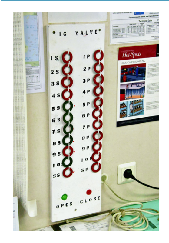
Figure 5: Marker board inert gas valves.
