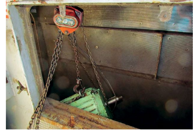
Fan duct and electromotor. (Source: Maersk)
