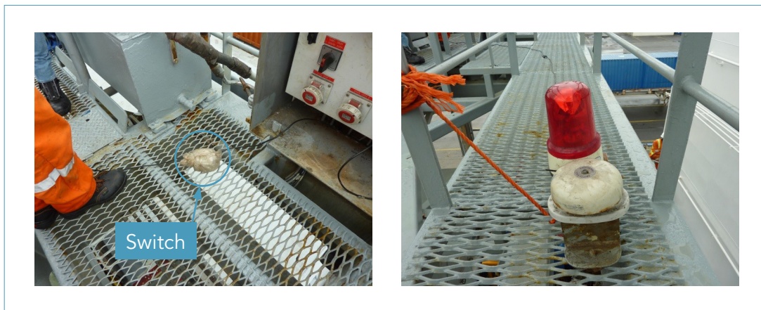
Alternative alarm system with on the left (figure 8) the switch and on the right (figure 9) the alarm bell and the strobe light.
