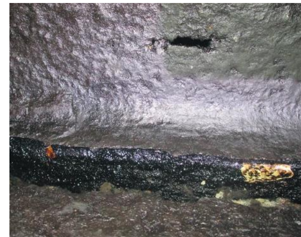
Crack in the bulkhead between the heavy oil tank and the ballast tank. (Photo: Iver Ships)
