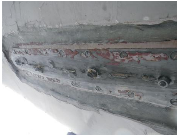
Broken-off keel bolts Capella. (Photo: Federal Bureau for the Investigation of Maritime Accidents)
