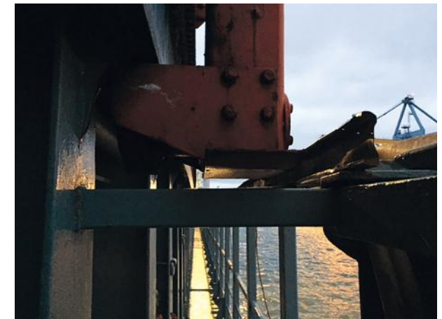
Location where the crew member must have become trapped. (Photo: Wijnne Barends)
