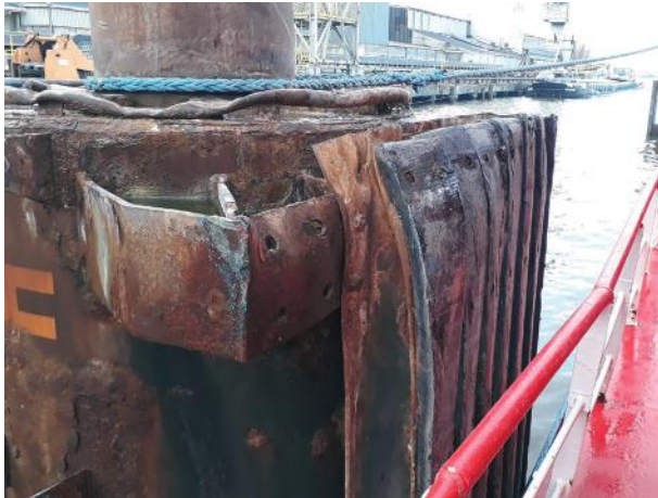
Damage to bollard and ship. (Photos: Human Environment and Transport Inspectorate)
