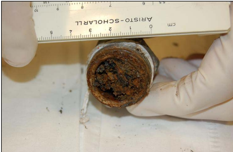
Figure 14: Blocked ventilation of the sewage tank (photo: TNO Construction and Service)
