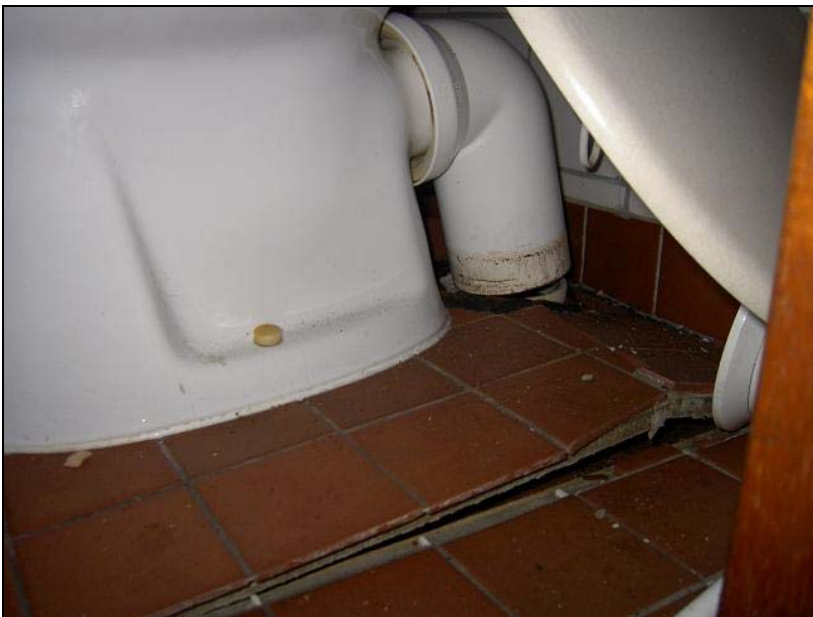
Figure 10: Toilet that had been fitted on top of the sewage tank. The way in which the floor has been forced upwards can clearly be seen. (photo: TNO Construction and Service)
