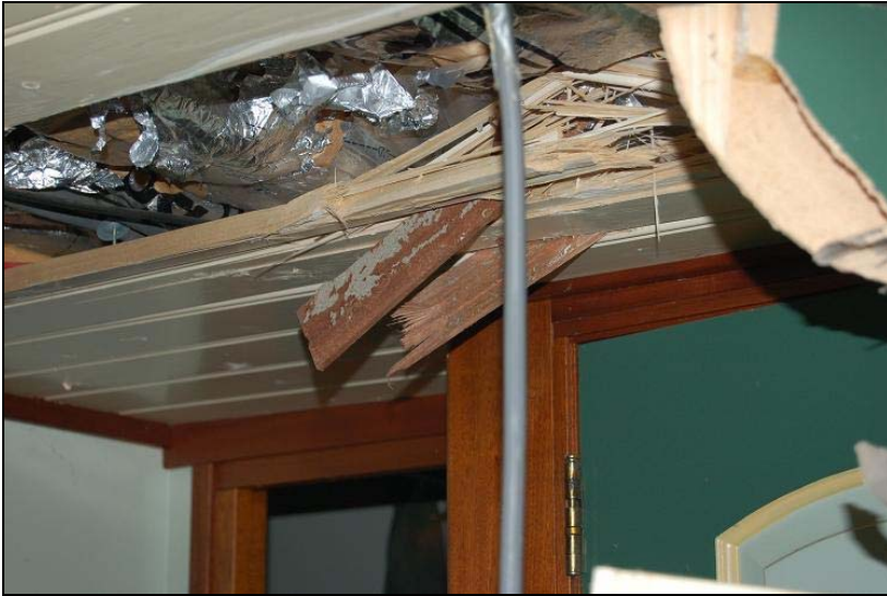
Figure 9: Damage to the ceiling. Parts of the laminated floor have bored themselves into the ceiling (photo: TNO Construction and Service)
