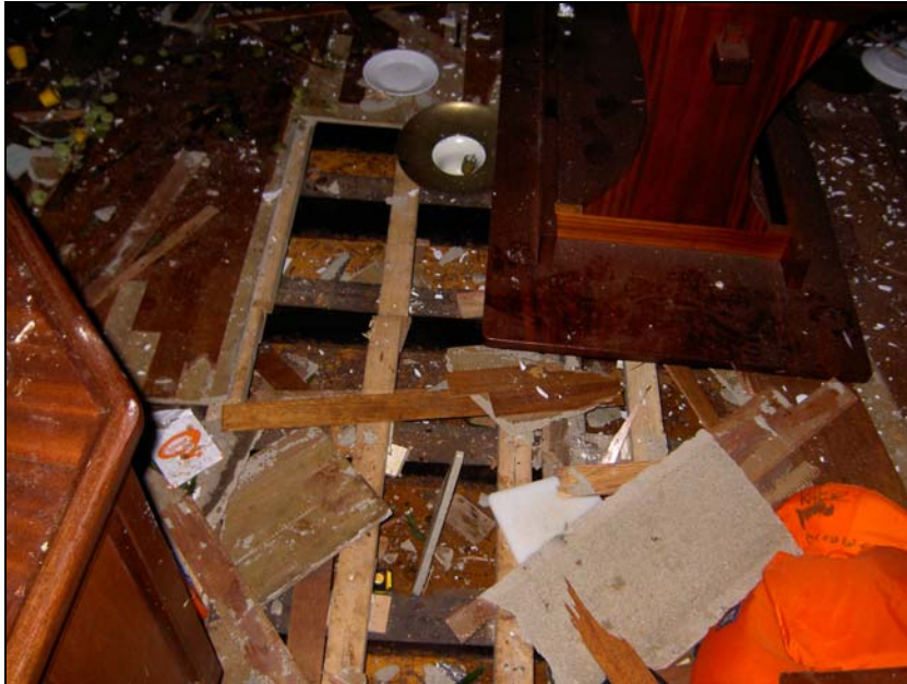
Figure 5: Damage after the explosion, floor of the living quarters (Photo: Dutch Safety Board).
