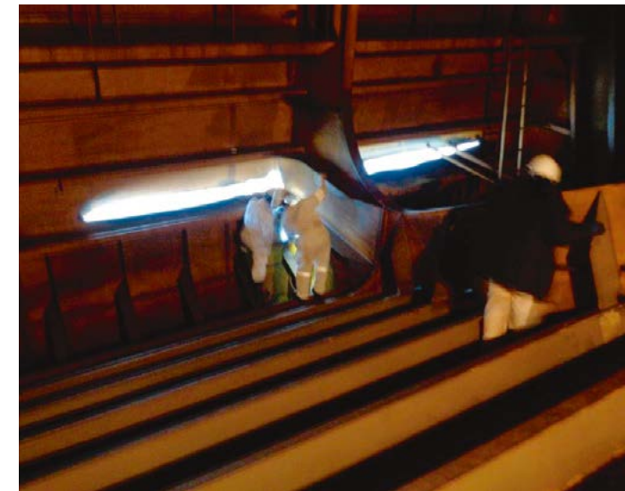
Breach in the stern of the Frontier Island. (Photo: Human Environment and Transport Inspectorate (ILT))
