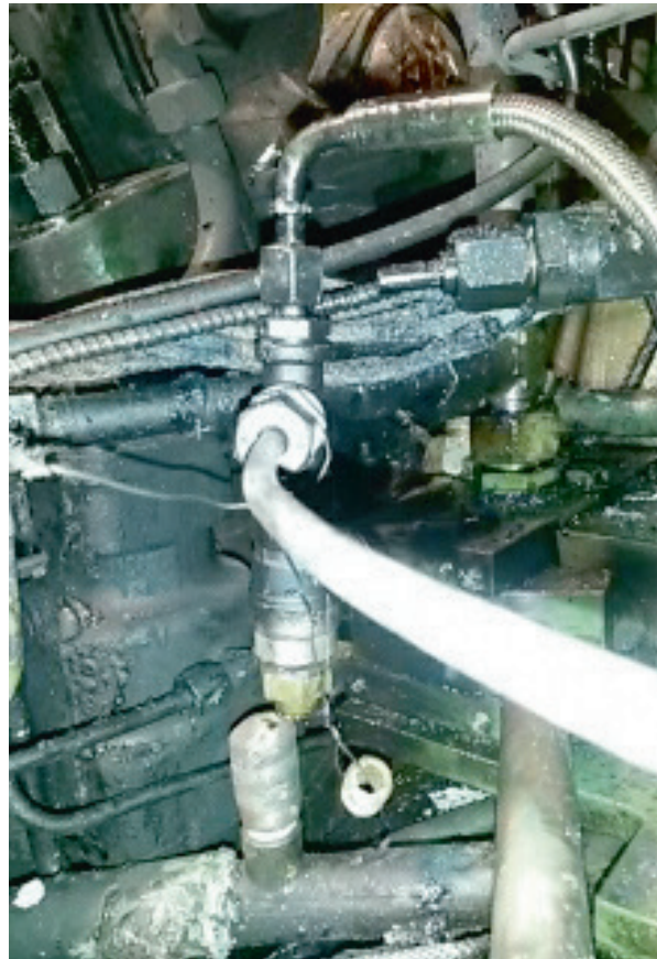
Broken fuel line.
