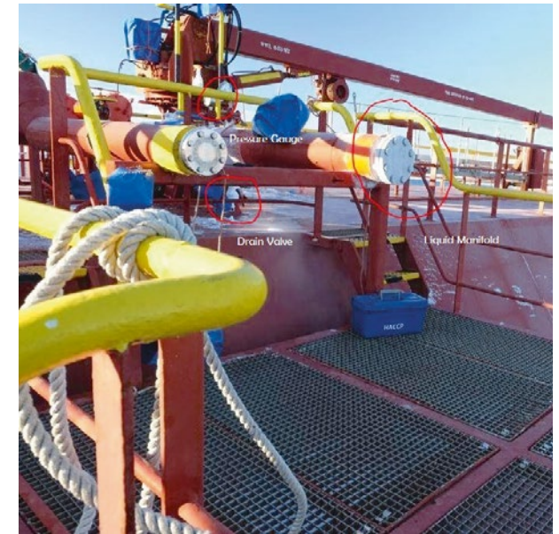
Location of the accident on the Coral Carbonic. (Photo: Antony Veder)
