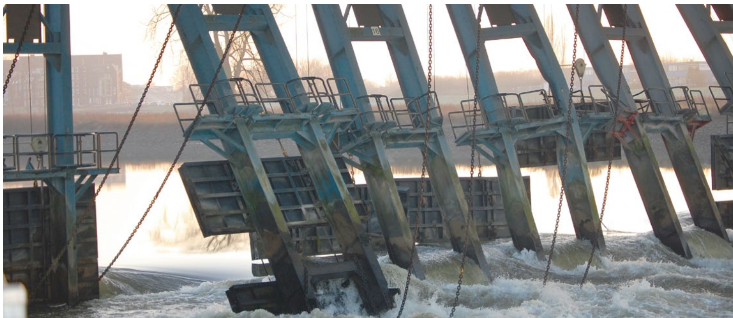
Damage to the weir at Grave after a collision by an inland vessel.
