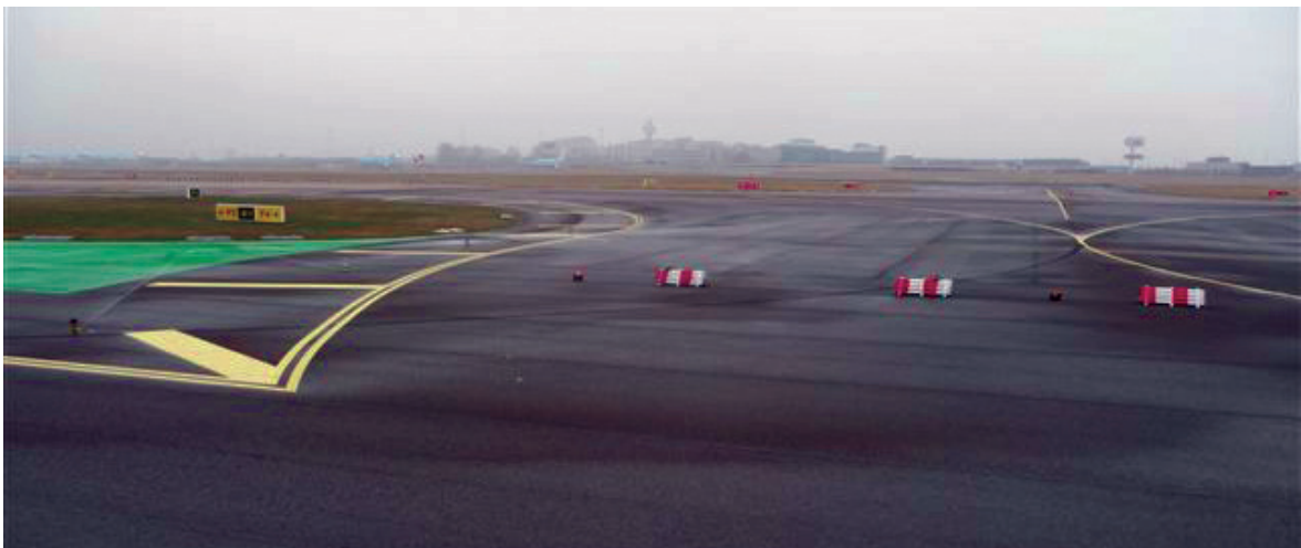
Figure 4: Intersection W11 (February 2013) looking from west to east (note the adapted lining and green painted surface as shown in figure 3, bottom drawing, infrastructural changes made by the airport authorities in June 2012).
