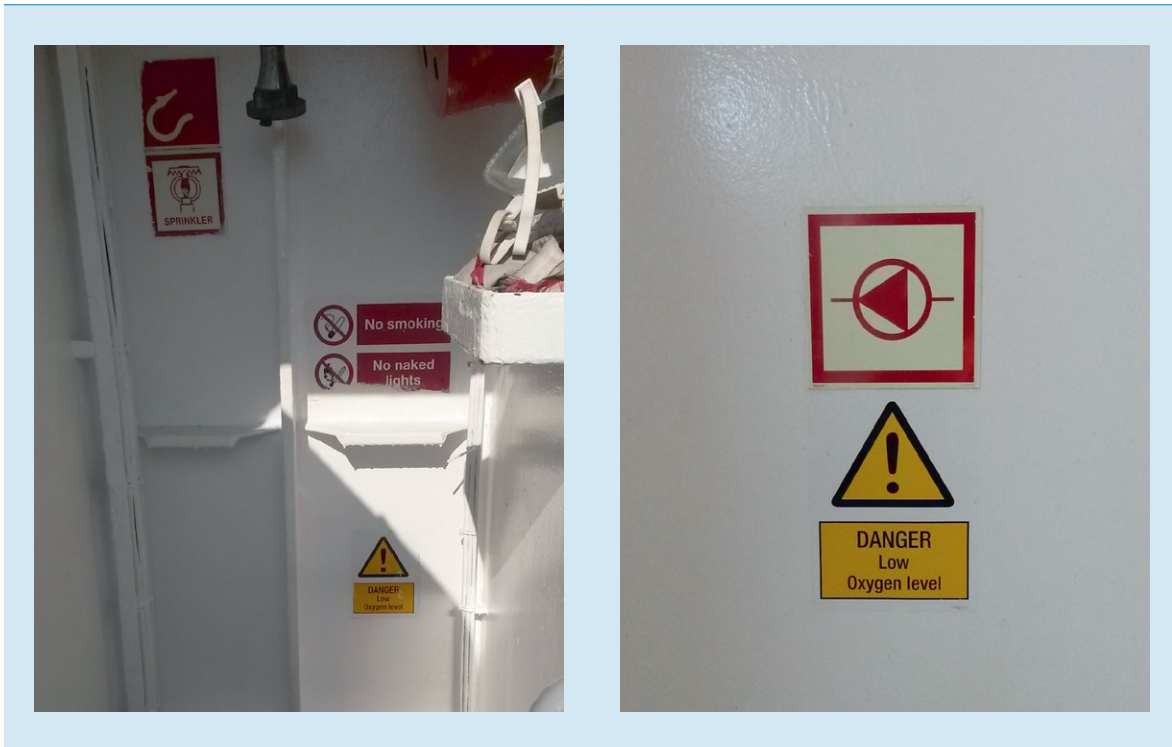
Figure 4: Warning stickers entrance to tank and bow thruster room. (Source: Wijnne Barends)
