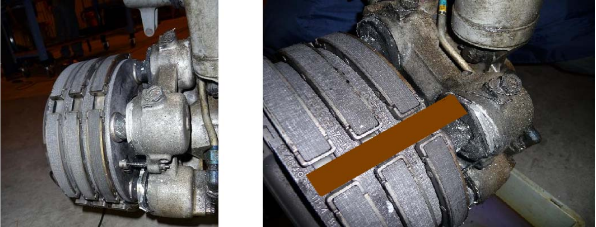
Figure 7: Brake cylinder damage on the left wheel strut with the brake discs on the left. On the right, the brown bar shows the position of the insert on the brake discs. The photograph shows that if the insert is able to move in a lateral direction, it can come into contact with the brake cylinders.
