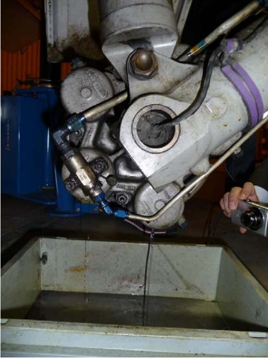
Figure 8: Detailed photograph showing the hydraulic fluid leaking from the two brake cylinders in the left wheel strut.
