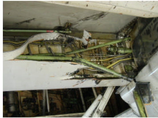
Illustration 2: Damaged parts of the flap system
