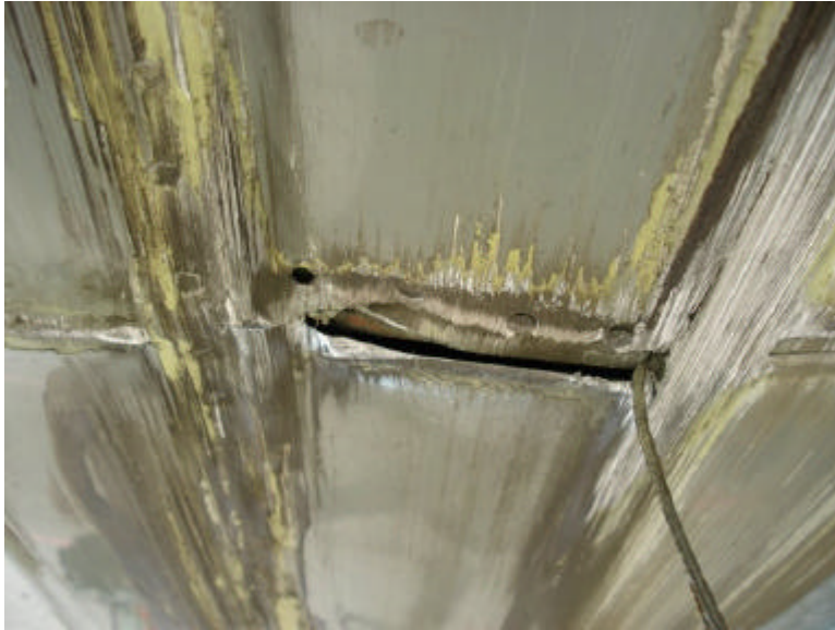
Figure 3: close up of the damaged area
