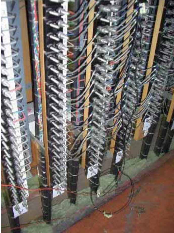
Illustration 2 The temporary connections are fitted in the relay housing using long black wires (Source of photo: Inspectorate for Transport, Public Works and Water Management).
