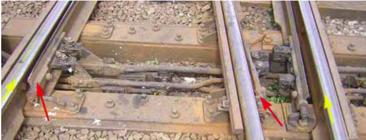
Illustration 3 Set of points 63B in the position found directly after the derailment. The open tongues can be clearly seen.
