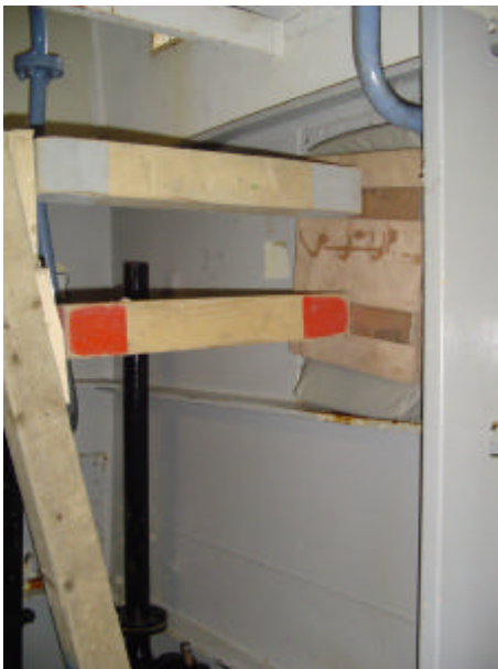
Illustration 2a. V-shoring against crack
