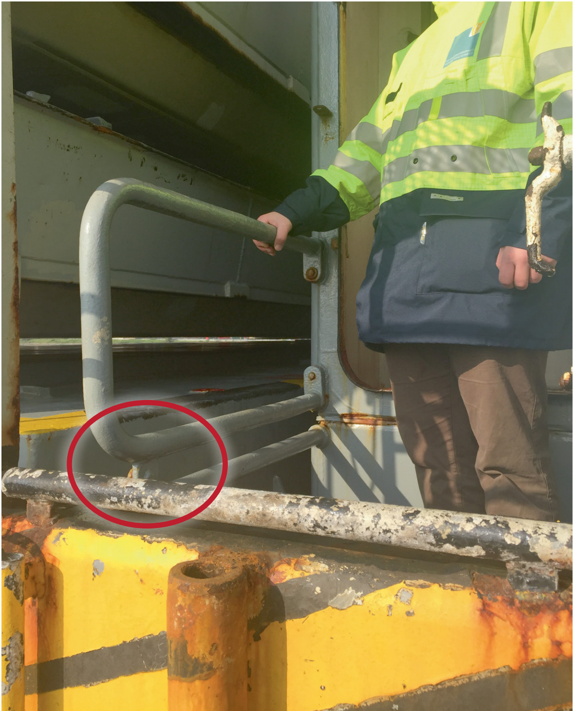
Figure 5: Site of the accident, hold access starboard portal amidships. (Photo: Dutch Safety Board)
