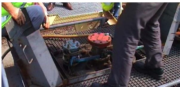
Fig. 6 Photograph of filler pipe (red) and return pipe (blue) and opened protective cover on top of the tank wagon, taken during testing following the incident (without acrylonitrile, i.e. without protective gas suits).
